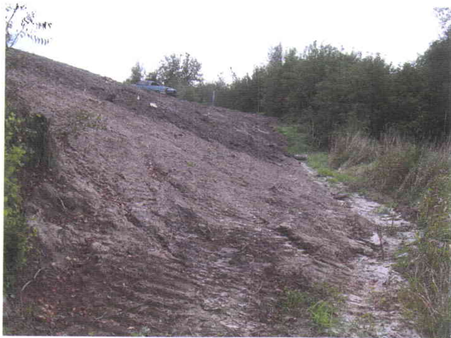
Photo 12 – Access to impoundment; wastes that were protruding through soil cover on eastern edge of Ravine No. 1 were covered; monitoring well G99-5 in the background (September 2004).
